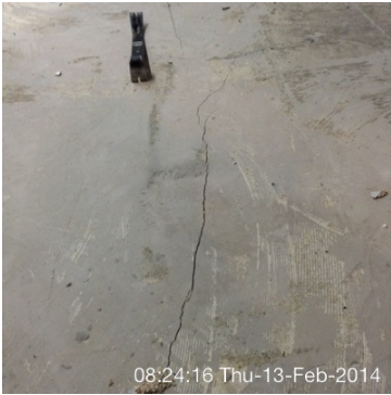
Crack by front entrance
