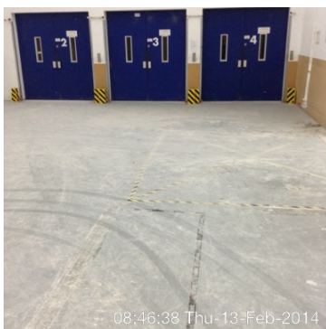
Resin by goods lifts
