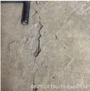
Crack over joint screed 10-15mm thick
